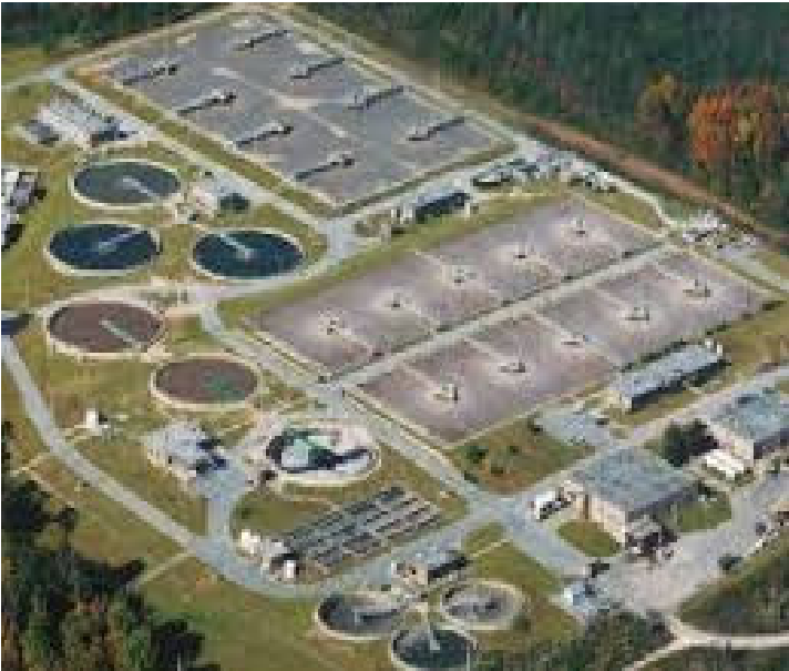
Lower Poplar Wastewater Reclamation Plant
